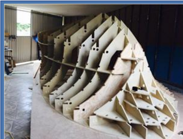
(C) The actual jig farming assembled on site and ready for the laminate inner hull core
