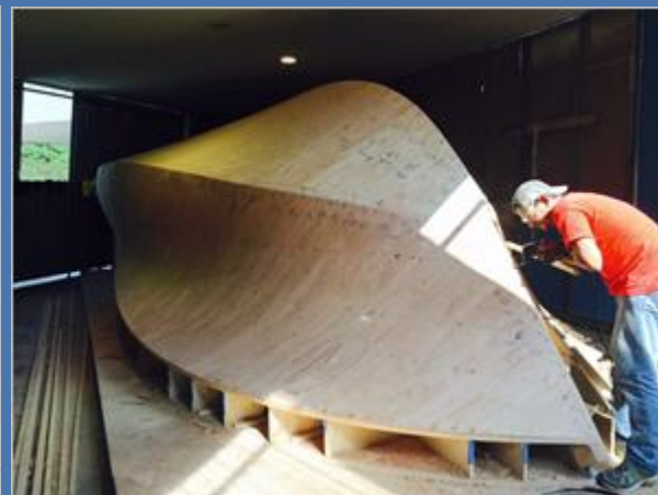
(D) The laminate inner hull core is complete and ready for the outer fiberglass hull
